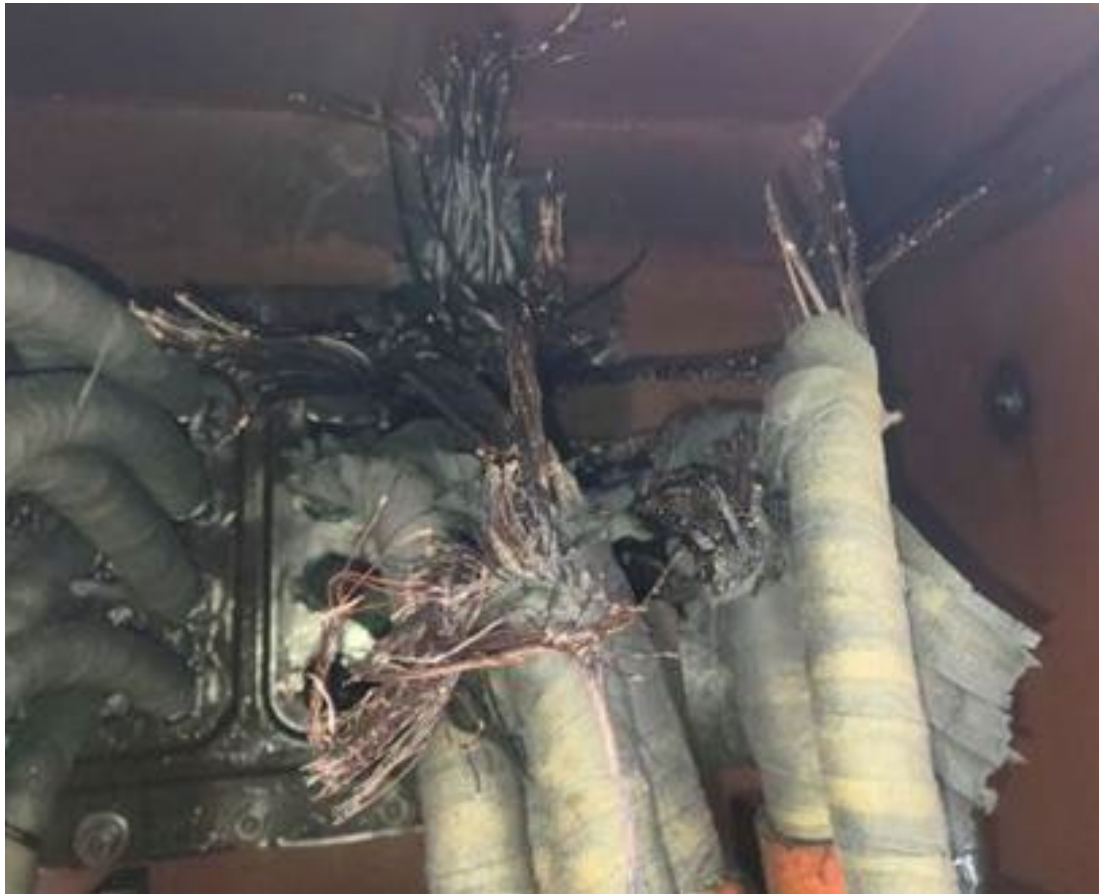
BULKHEAD TAP BOARD AND TAP CABLES
