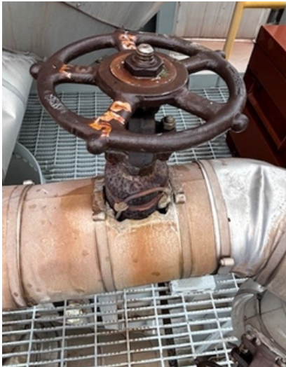
Valve stem without insulation
