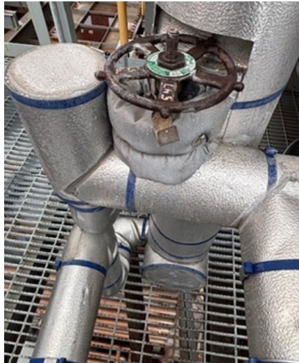
Valve stem with insulation
