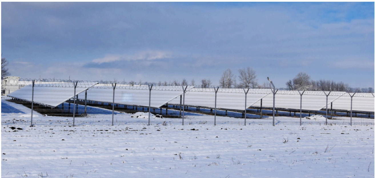
Solar panels secured behind fenced area
