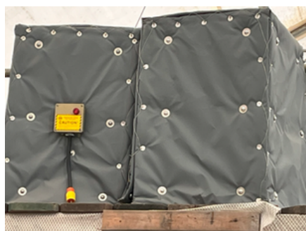
Portable "hot boxes", powered by 110 VAC, used to address freezing issues for instrumentation not permanently protected
