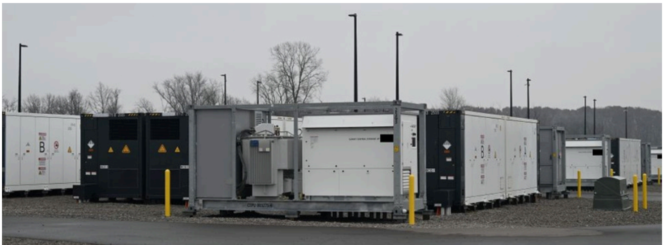
Battery storage pods with inverter in front
