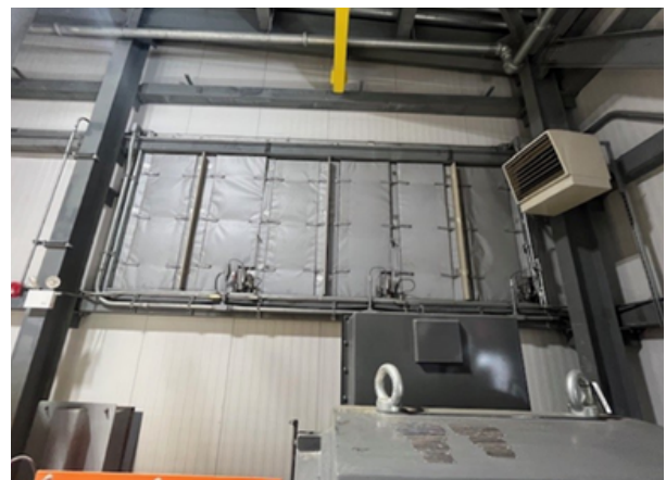
Removable insulation covers overbuilding louvers
