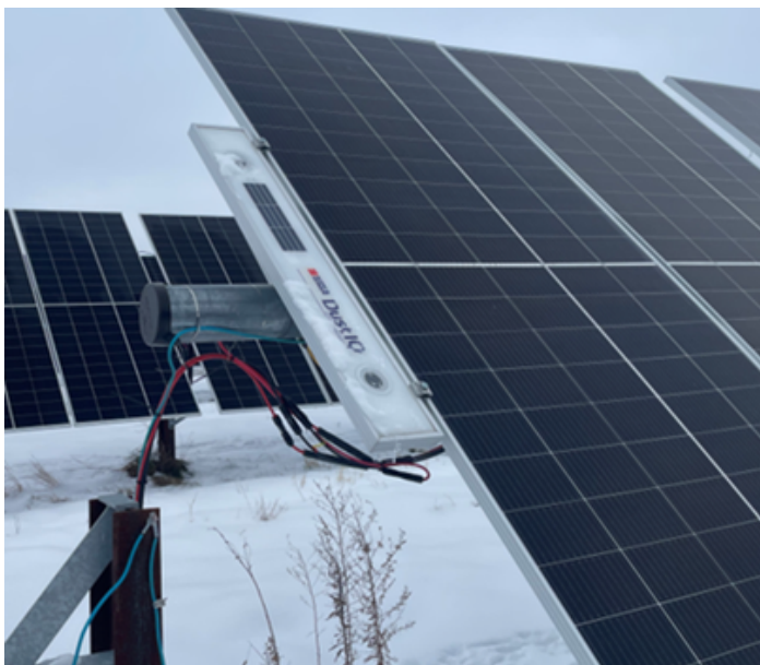
Dust monitoring system
