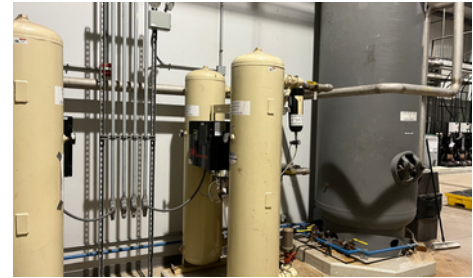
Compressed air supply system
