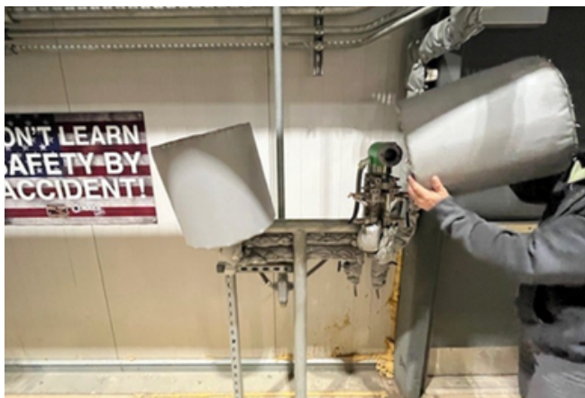
Insulation covers for transmitters and sensing lines indoors but located near an external wall/door
