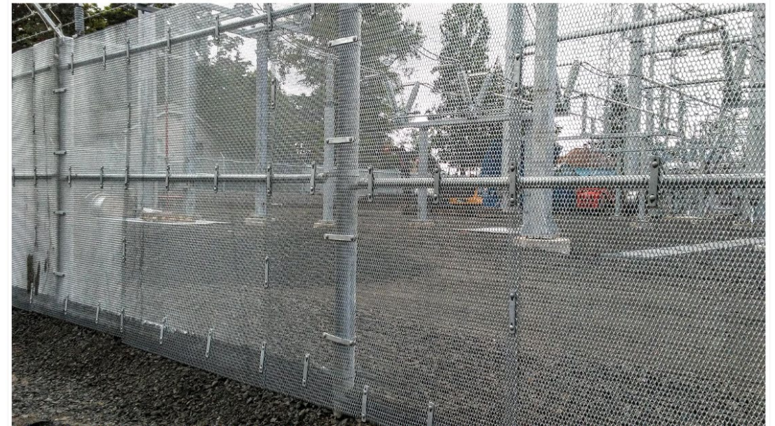
The metal fence around Pacific Power's expanded Hazelwood substation on Southwest 17th Avenue.
